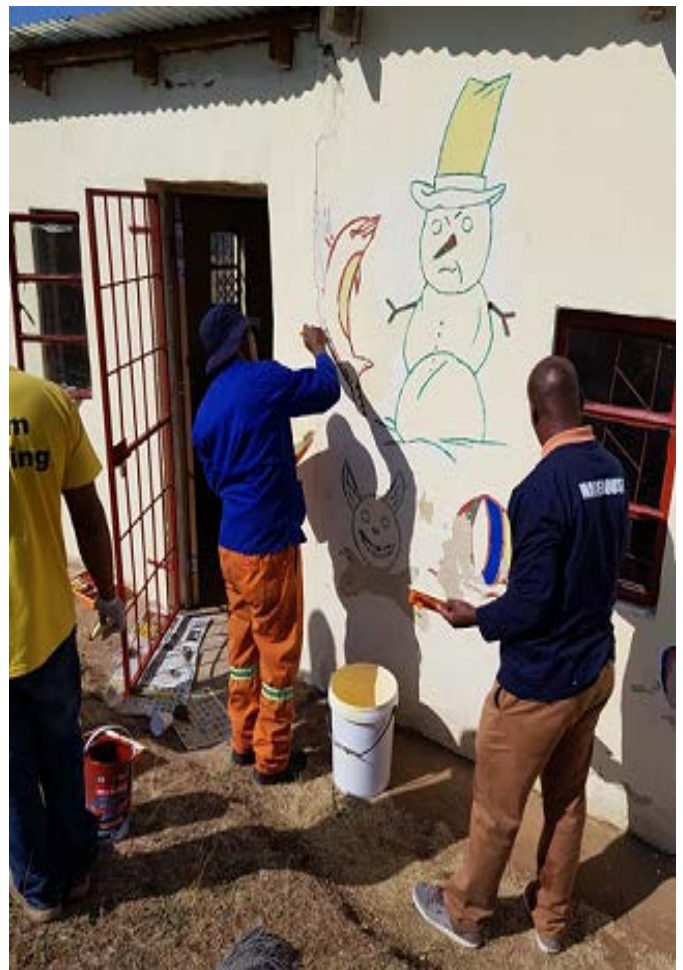
Pic 3a. Shu Powders employees putting the final touches on the paint work.
